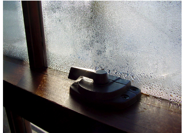
Window condensation of this level promotes the growth of mold and mildew, and indicates lower-than-ideal indoor air quality. Photo credit: Steve Maxwell
