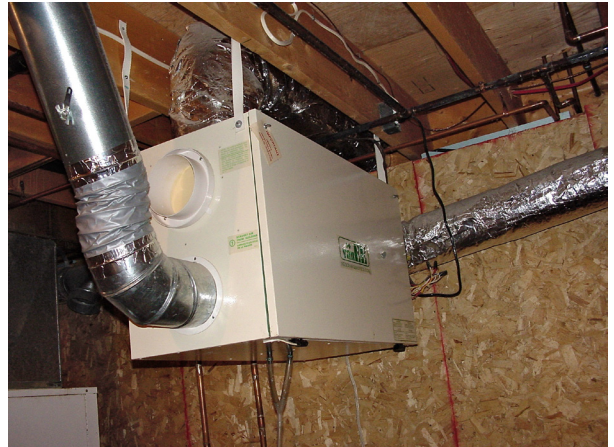
All heat recovery ventilators look similar. This unit is hanging from basement ceiling joists, connected to the outdoors by two ventilation pipes. One draws fresh air in, and the other exhausts stale air outside. Photo credit: Steve Maxwell
