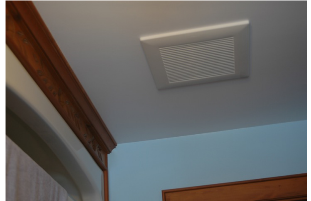
This high-capacity exhaust fan was retrofitted into a bathroom that didn't have a fan before. It moves 150 cubic feet of air per minute, and is located just outside the shower so it can capture and remove moisture quickly. Photo credit: Steve Maxwell
