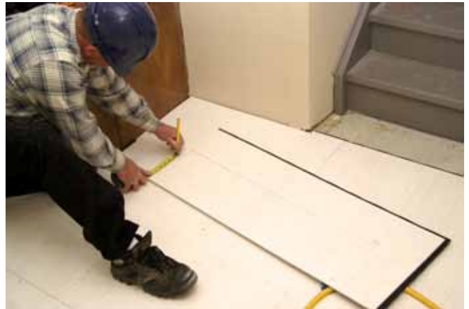
A moisture and mold-resistant subfloor may be the single most important feature in any basement finishing campaign. Here a subfloor product is being marked for cutting before installation over a concrete basement floor. Photo credit: Steve Maxwell
