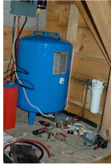
This 12-volt DC water system delivers pressurized water using power stored in a battery by PV panels.
