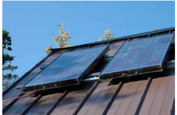
These rooftop PV panels generate power for a water system and lighting at a lakeside cottage many miles from the power grid.
